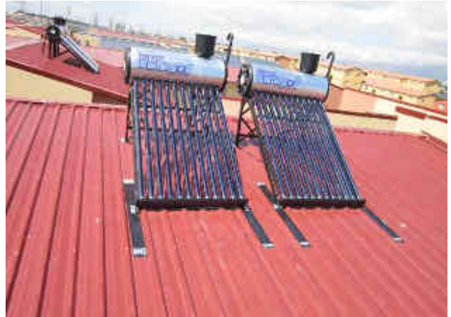
Figure 8: Solar water heaters at Joe Slovo, showing different orientation of units
